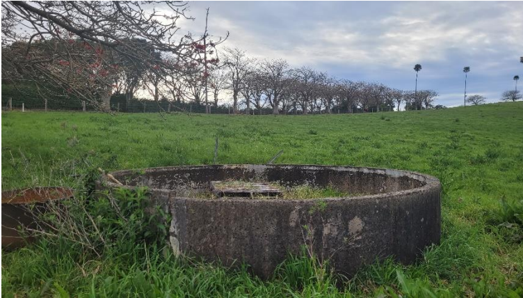
Photo 47 North-east facing view of a concrete tank in the far southern portion of the study area
