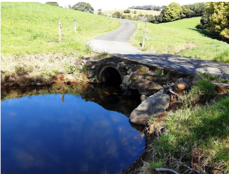
Photo 48 South facing view of a bridge and culvert over Spring Creek on the driveway to the northern homestead complex
